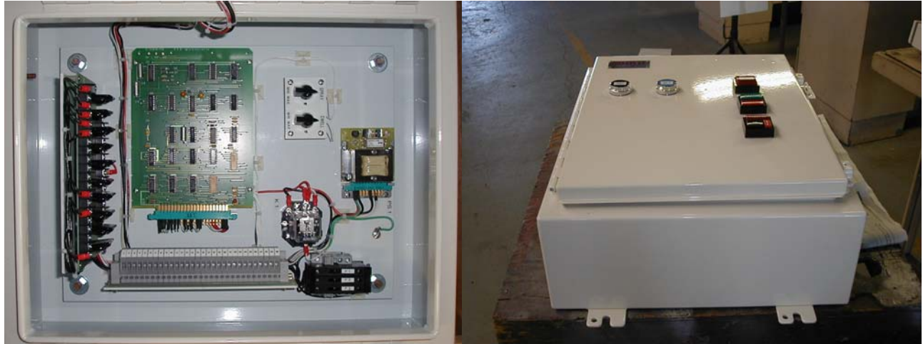
Figure 4 - Marker Control Enclosure
